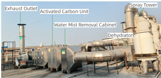
Upgraded Waste Gas Treatment System
