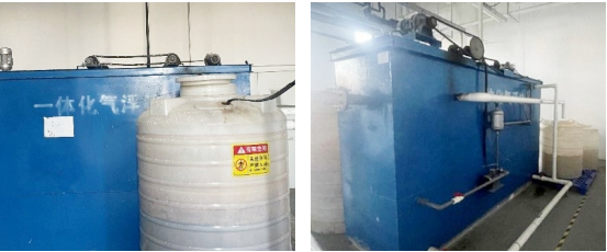
Wastewater Treatment Facility at Jiangmen Base
